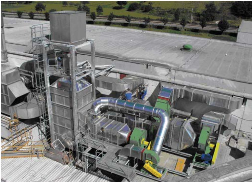
Modernization of the waste air recovery system
