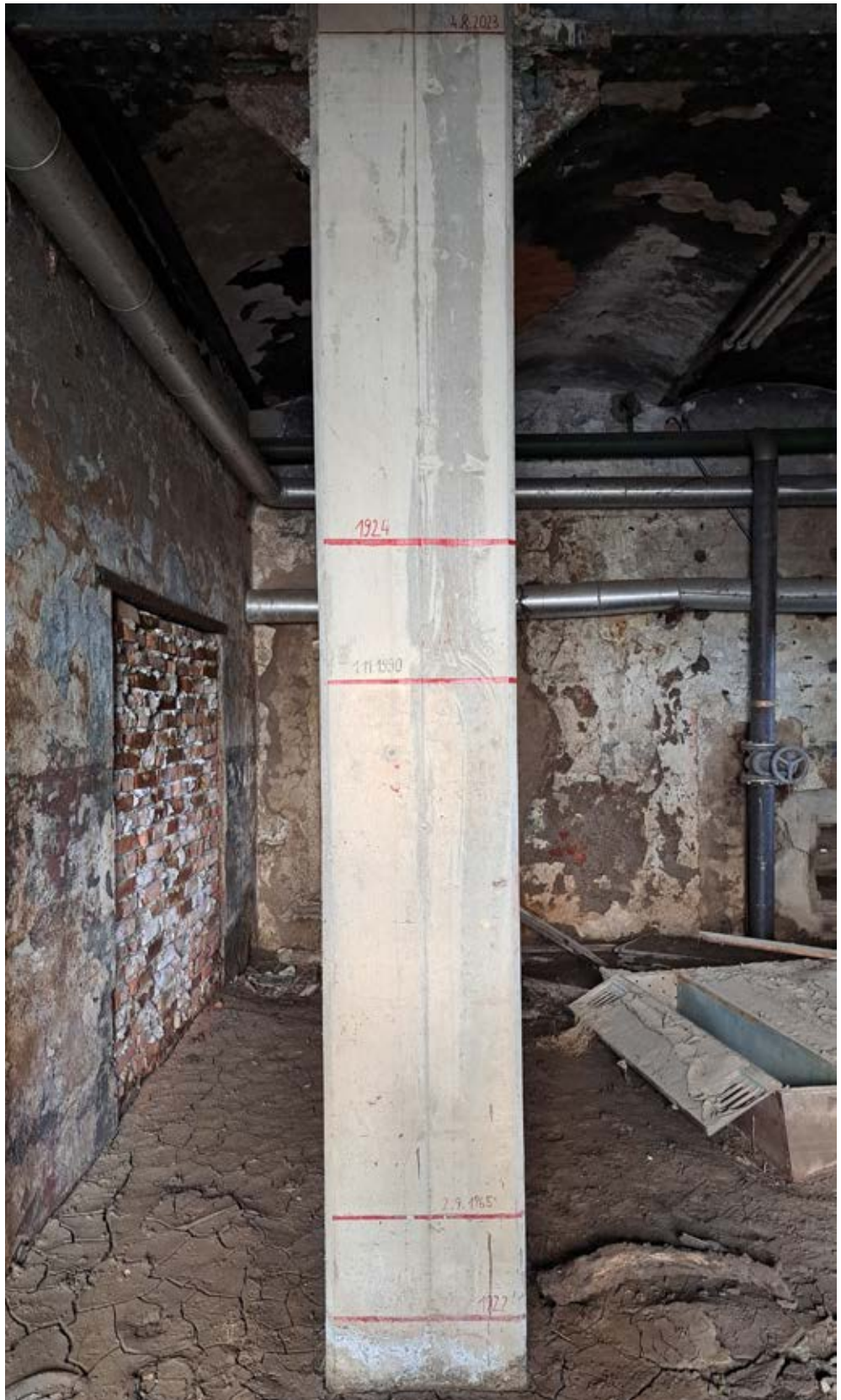
Column marking flood levels. August 4 th 2023 – highest level.
