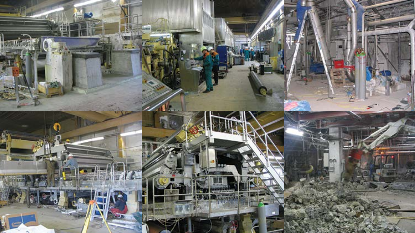
Paper machine during renovation in 2006
